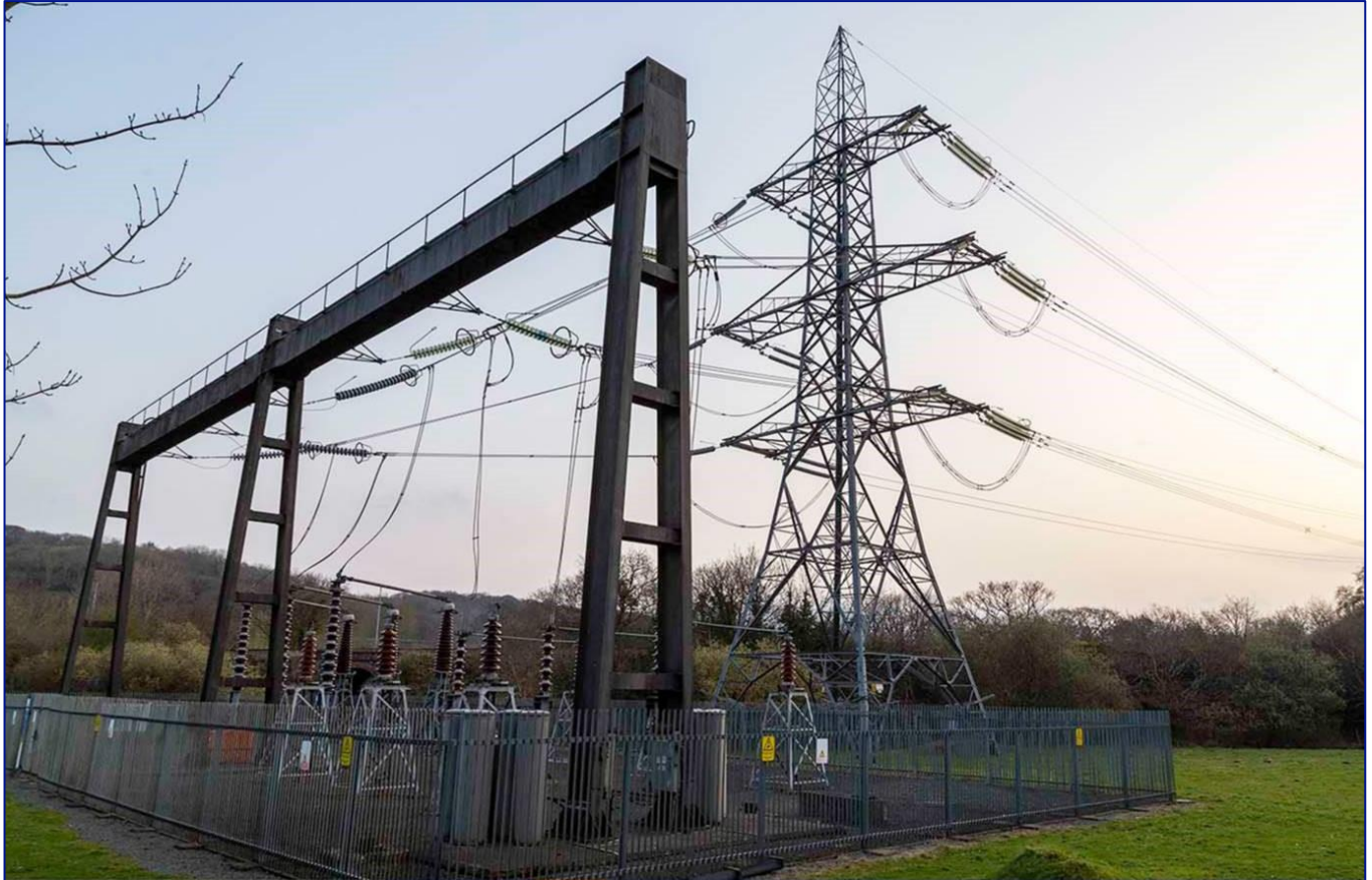
Photograph 4.6 – Typical Cable Sealing End Compound
