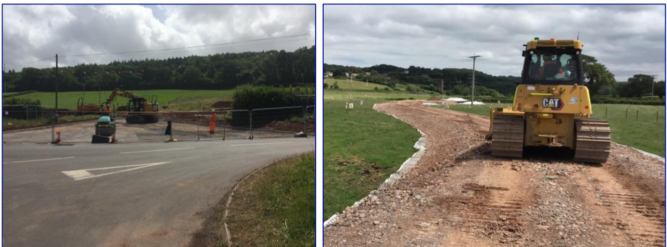
Photograph 4.1a – Construction of a Bellmouth and 4.1b – Example of Temporary Access Route Made of Imported Stone
